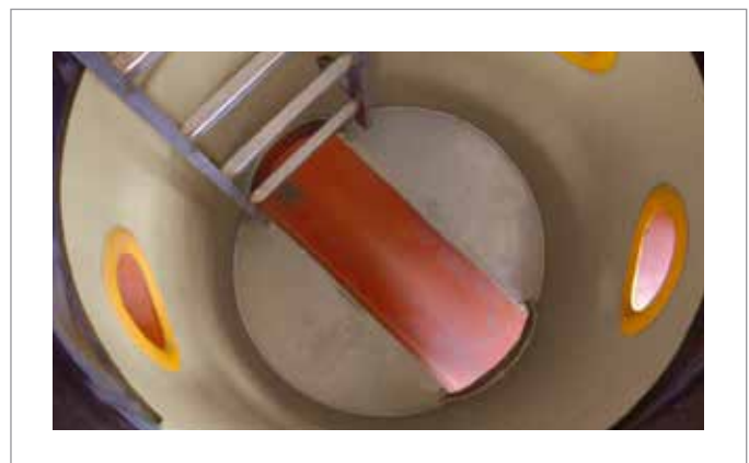
Seen from the inside of an inspection well, in one of the multiplicity of possible configurations.
